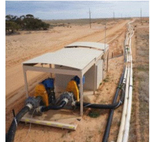
Slurry Booster Stations & pipelines
