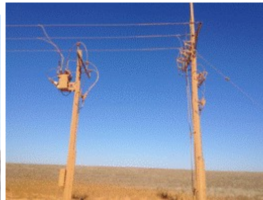
Power poles, wires & transformers
