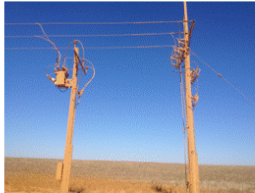
Power poles, wires & transformers
