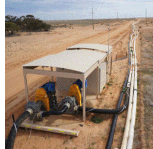
Slurry Booster Stations & pipelines
