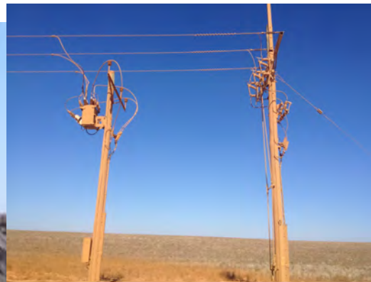
Power poles, wires & transformers
