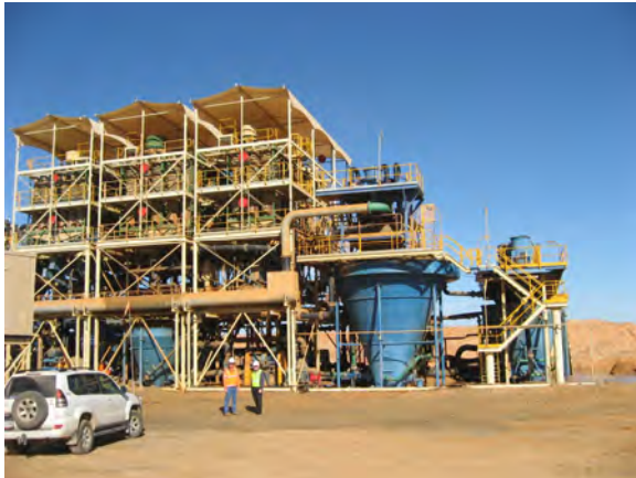
Wet Concentration Plant
