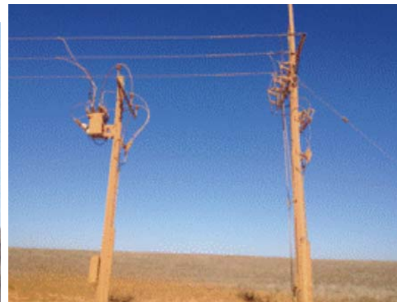
Power poles, wires & transformers
