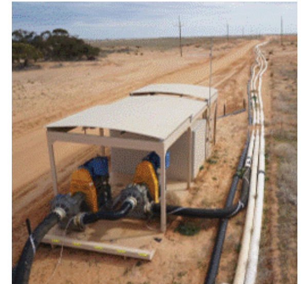
Slurry Booster Stations & pipelines
