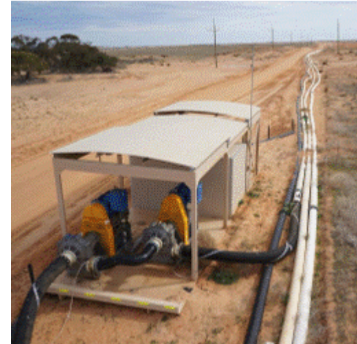
Slurry Booster Stations & pipelines
