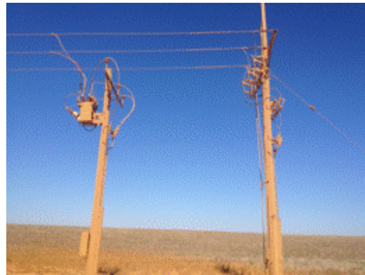
Power poles, wires & transformers
