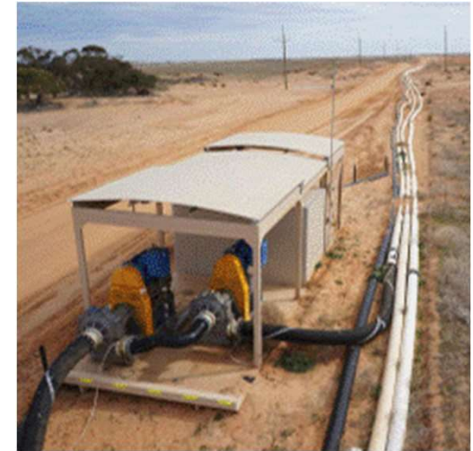
Slurry Booster Stations & pipelines
