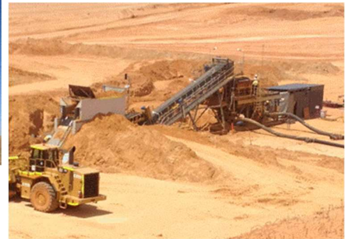
Mine Slurry Unit
