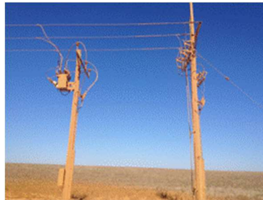
Power poles, wires & transformers
