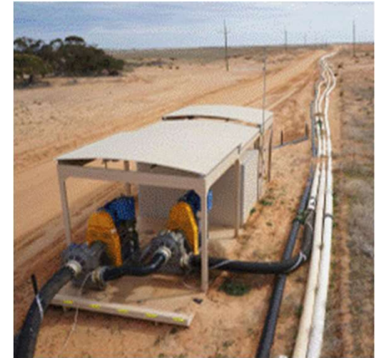
Slurry Booster Stations & pipelines
