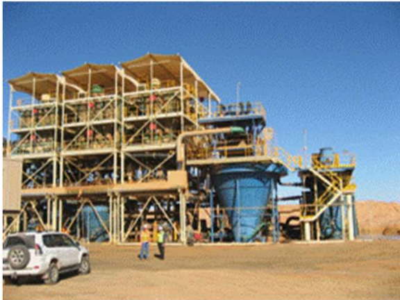
Wet Concentration Plant
