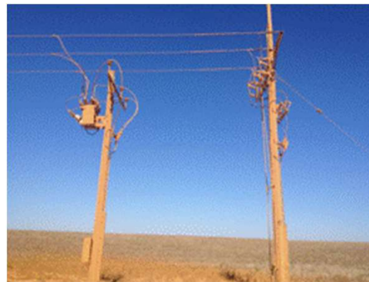
Power poles, wires & transformers
