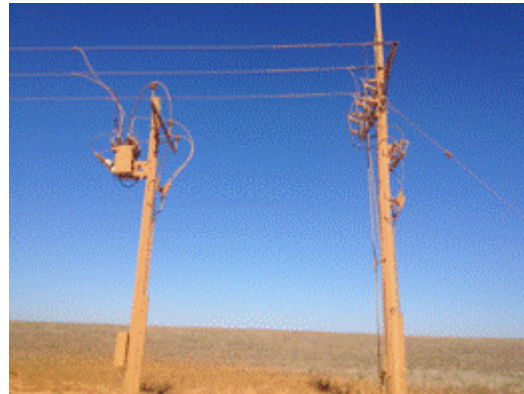
Power poles, wires & transformers
