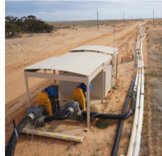
Slurry Booster Stations & pipelines
