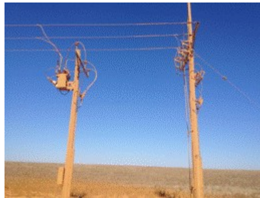
Power poles, wires & transformers
